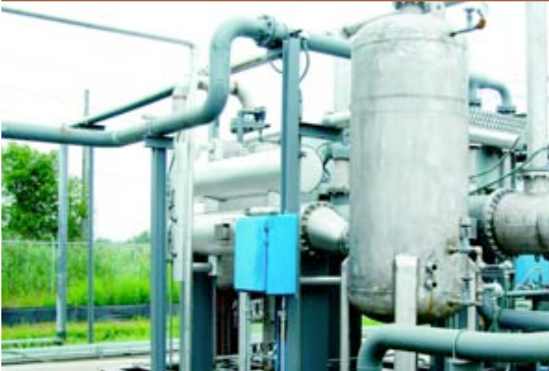
DSWA's gas collection contractor, Cereza, collects landfill gas and prepares it for transport to the nearby Connectiv plant.
